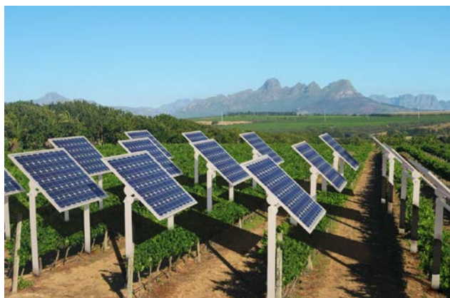
Fig. 10. Solar panels over vineyards.
